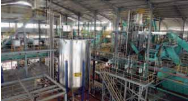
Zero water dilution system to minimise waste generation at Genting Jambongan Oil Mill
