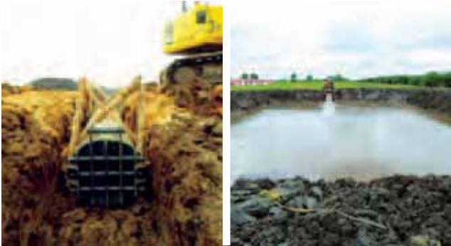
Water management using flood gates (left) and perimeter bunding with retention pond (right)
