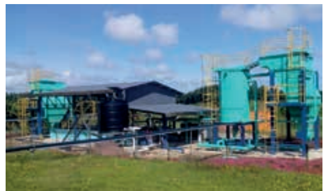
Bioflow and membrane bioreactor plant at Genting Mewah Oil Mill
