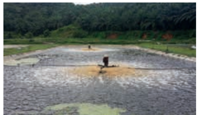
Mixers and aerators installed in effluent ponds
